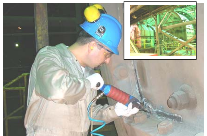
Figure 11. Application of UP for rehabilitation and repair of welded elements of mining equipment
