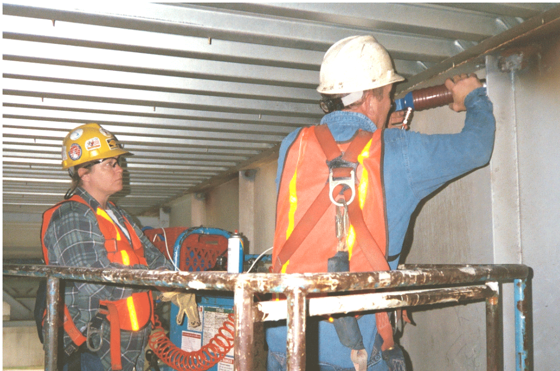
Figure 9. Ultrasonic Peening of welded bridge: UP of the end of one of welded vertical stiffeners
