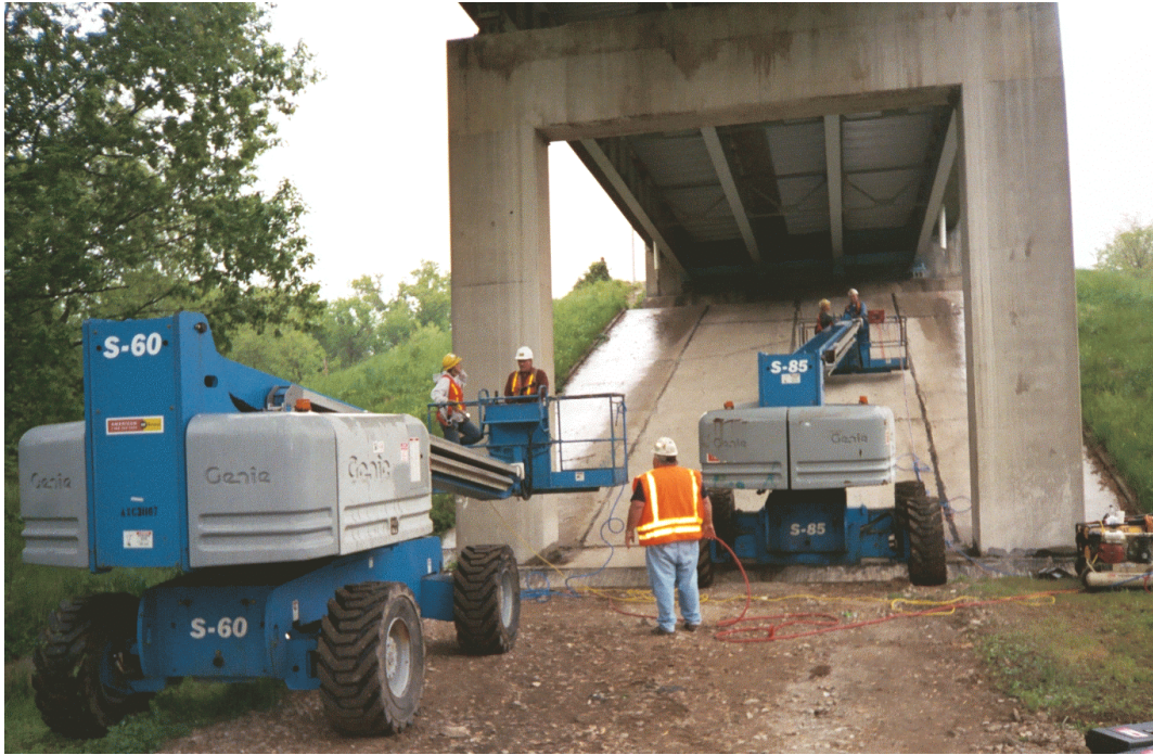
Figure 8. Ultrasonic Peening of welded Bridge: Preparation for UP treatment (Two UP Systems/Lifts)
