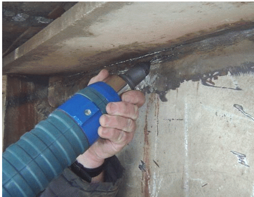
Figure 11. Enlarged view of the zone of repair (welding +UP treatment) of fatigue crack in welded element of bridge span.
